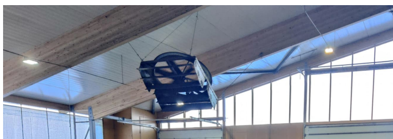
Figure 5. Example of a large fan mixing the air inside the Arvela barn.
